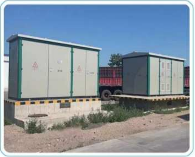
Construction Project of Supporting Engineering for Xinxin Nengke Xingtai Power Exchange Station
