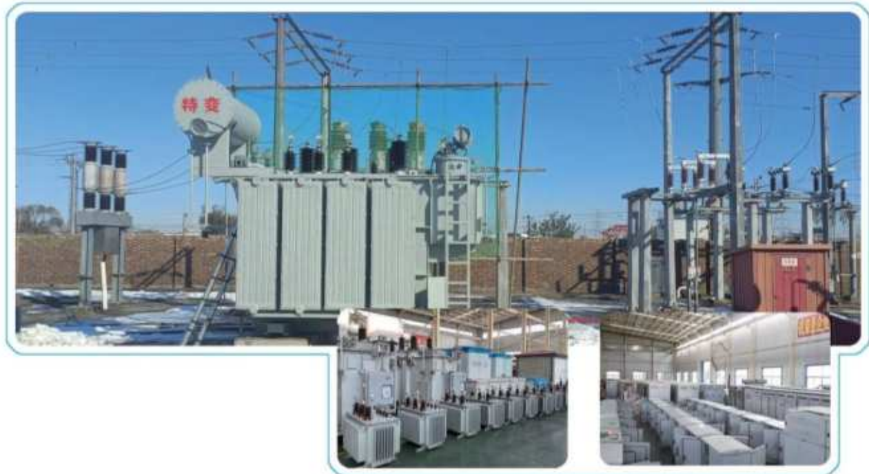
Procurement Project of 35KV Main Transformer, Box type Substation, 10KV Transformer and Distribution Cabinet for Huanghua Coal to Electricity Project
