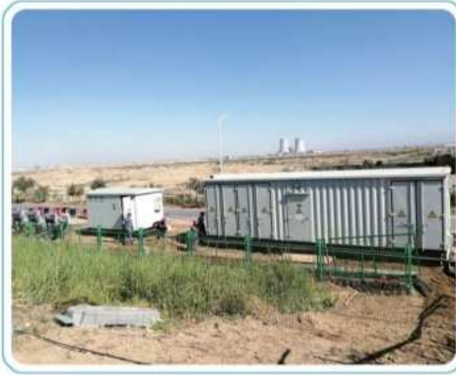
Xinjiang Oriental Hope Nonferrous Metals Co., Ltd. 300000 m 3 Water Tank Distributed Photovoltaic Project Prefabricated Cabin and 3150kVA Box Transformer Procurement Project
