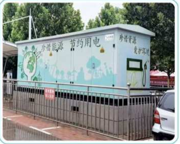
Shanxi Xiangfen Supermarket 10KV Charging Pile Project
