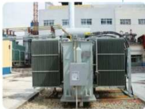
35kV Power transformer with OLTC
