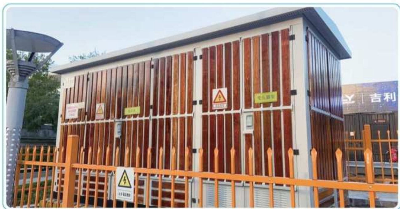
Geely Group Yiyi Interconnected Box type Converter Station Project
