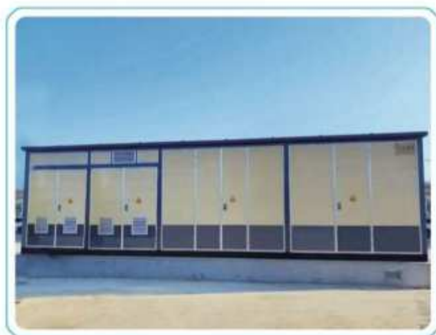
The 35KVA project of Ningde Times Weiqiao Power Exchange Station in Zouping City
