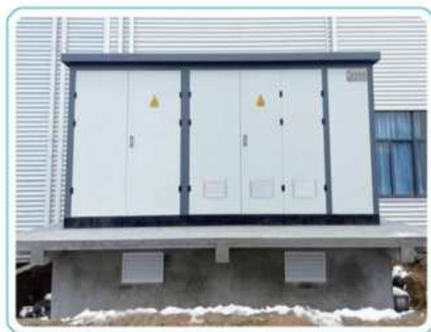
13.8 MW Distributed Photovoltaic Power Generation Project in Zhongding Industrial Park, Zhongde Intelligent Manufacturing Town, Ningguo, Anhui Province
