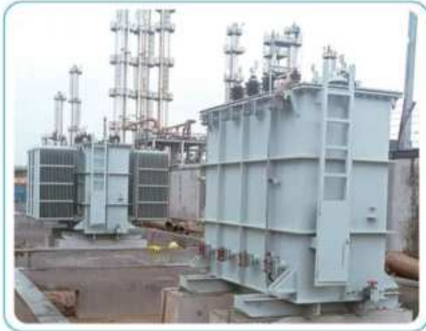
Dongying Wanda Group S20- 12500KVA/10.5kV
