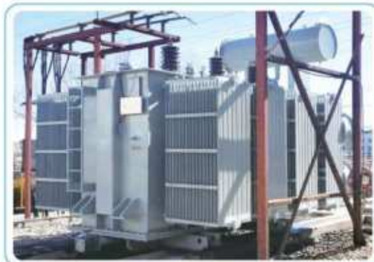
SZ20-16000KVA/35kV Transformer Procurement Project of Tianyuyuan New Energy Co., Ltd. in Bayannur City, Urad Front Banner, Inner Mongolia
