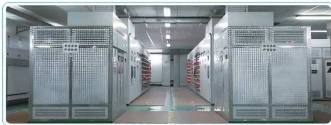
Installation project of 20 dry-type transformers for Qingdao Dayungu Jinmaofu residential area supporting projectTransformer Procurement ProjectProject
