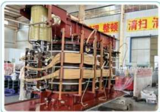
Disassembly Test Project of 110kV Fault Transformer of Institute of Electrical Engineering, Chinese Academy of Sciences
